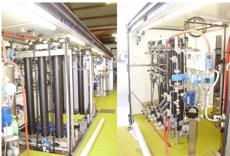
Figure 1 – PhosEnergy Process Demonstration Plant
