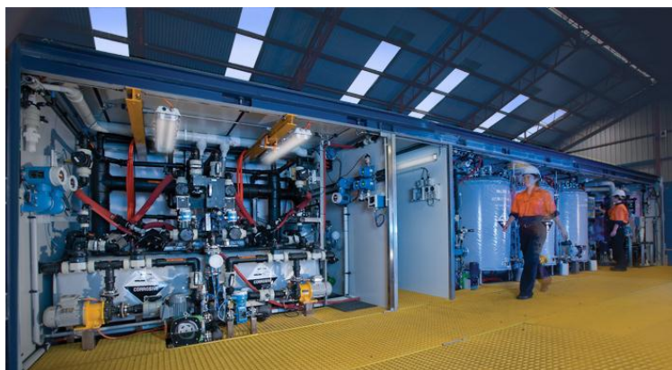
Figure 7 – PhosEnergy Process Demonstration Plant
