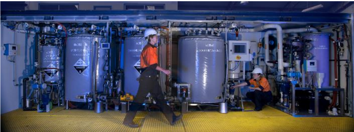
Figure 1 – The PhosEnergy Demonstration Plant
