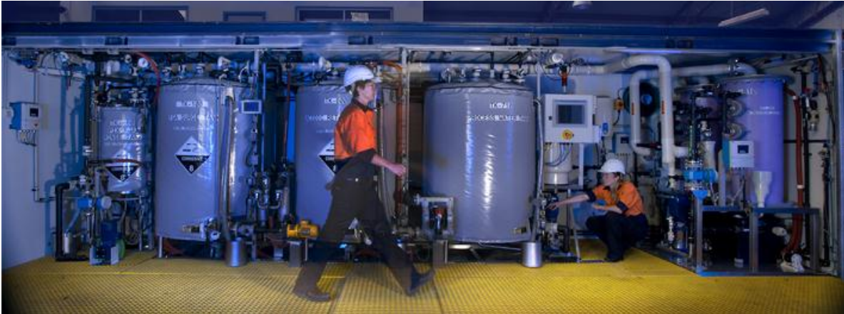
Figure 1 – The PhosEnergy Demonstration Plant
